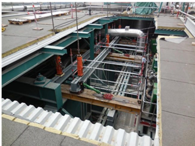
Figure 14. The roof of the boiler has been opened and front wall is being pushed outwards using hydraulics.
