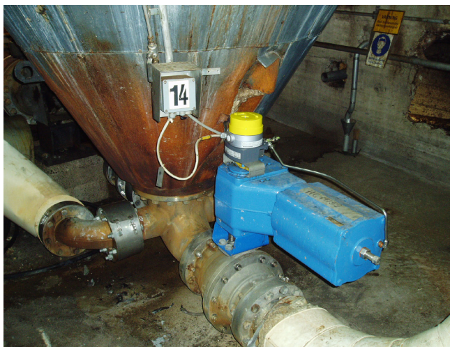
Fig. 4. SwitchGuard and blow valve after the digester
