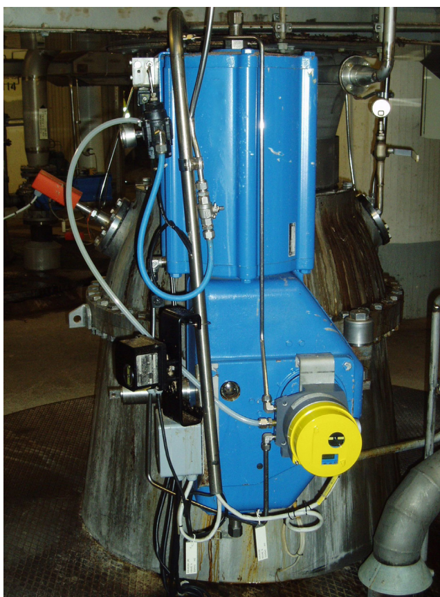
Fig. 3. SwitchGuard and capping valve atop the digester
