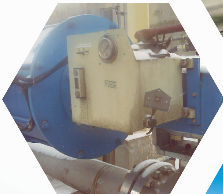
Installation at - 45 °C, Upper Mongolia, (Installed since 2006)
