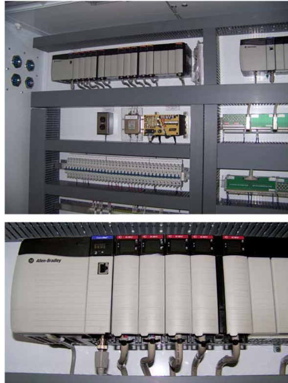
Figure 3. This pre-assembled PLC cabinet (top), featuring Allen-Bradley ControlLogix PLC (bottom), controls a soft calender, and will be pre-installed in the mill's MCC room.
