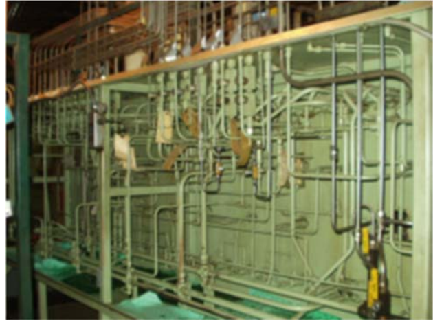
Figure 9. The original valve panel included obsolete, hard-to-find parts and lacked modern safety controls.
