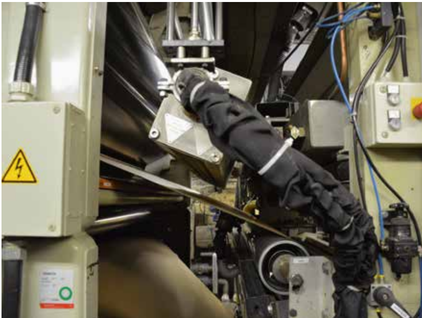
ONE OF TWO IQ MOISTURIZER SPRAYBOOMS INSTALLED ON THE CORRUGATOR.
