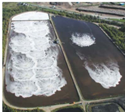
Figure 1. Aerated basin secondary effluent treatment
